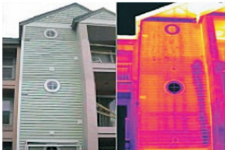
Upper unit laundry room water leak behind the siding
